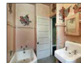
bad point: bathroom condition
